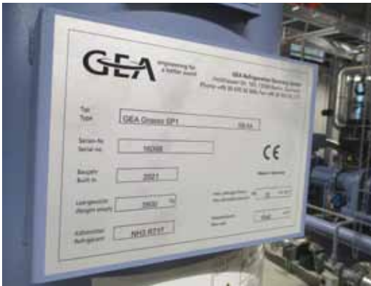
➤ Type plate from one of 3 compressor packages
