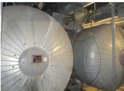
➤ Refrigerant separator of the existing system
